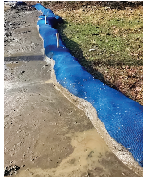
Figure 1: 8-inch Compost Filter Sock
